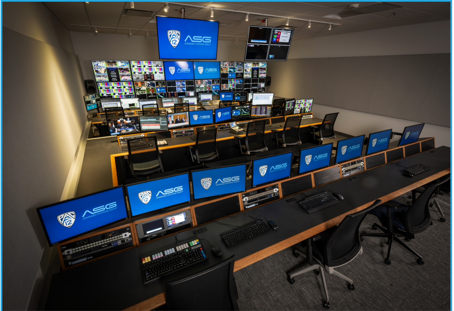
Pac-12 Networks Production Control Room 1
