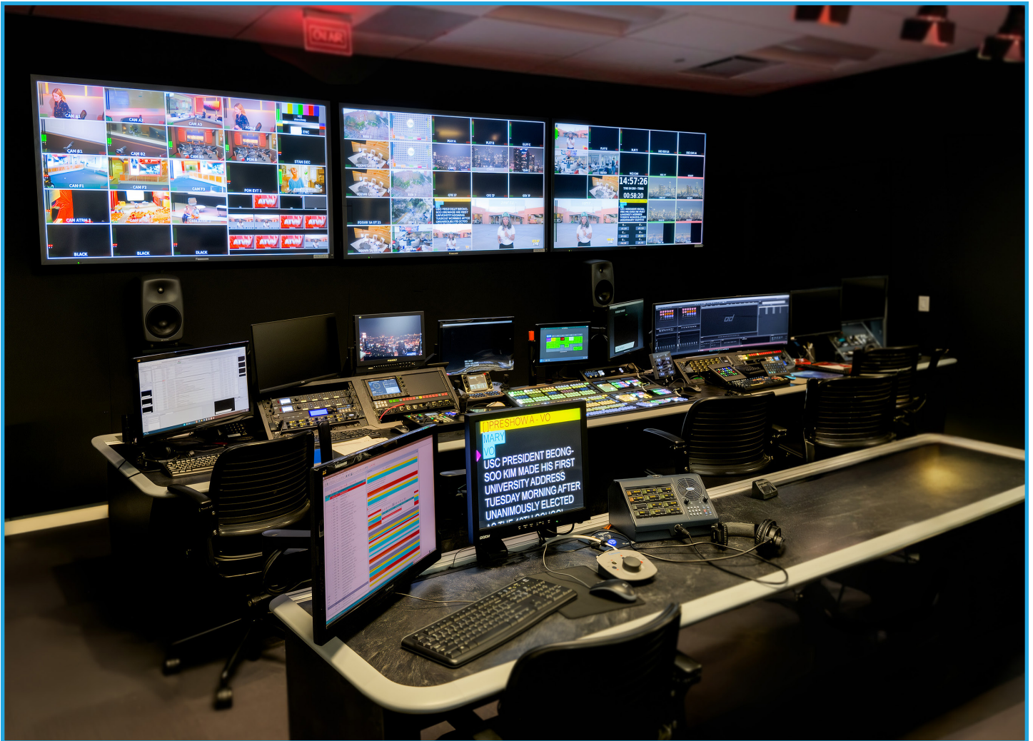
Studio C Control Room
