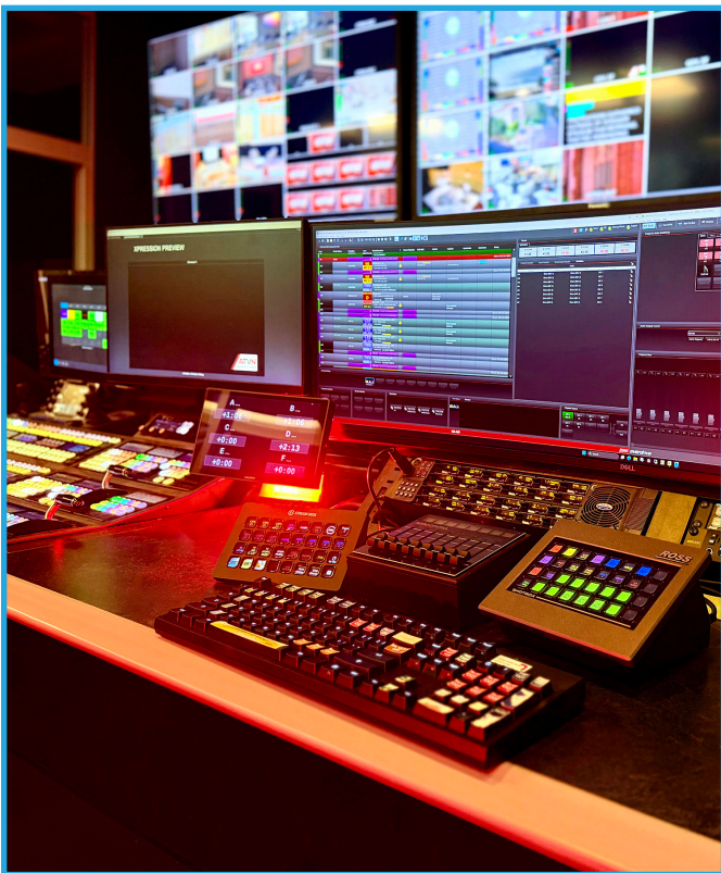
Studio C Control Room
