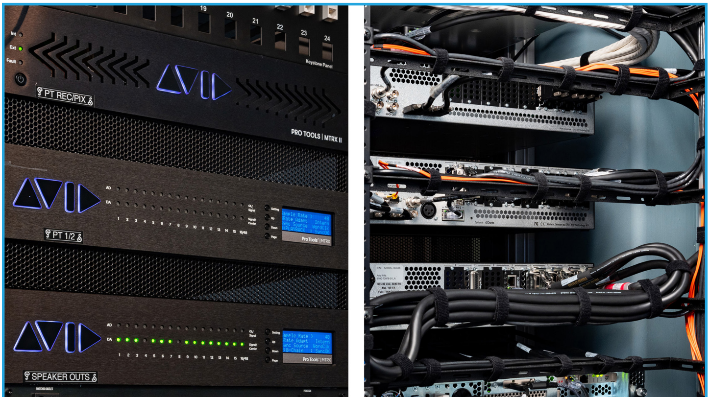
Front and back of gear rack in the machine room of Evergreen Studios. Photos by MixBus Marketing.
